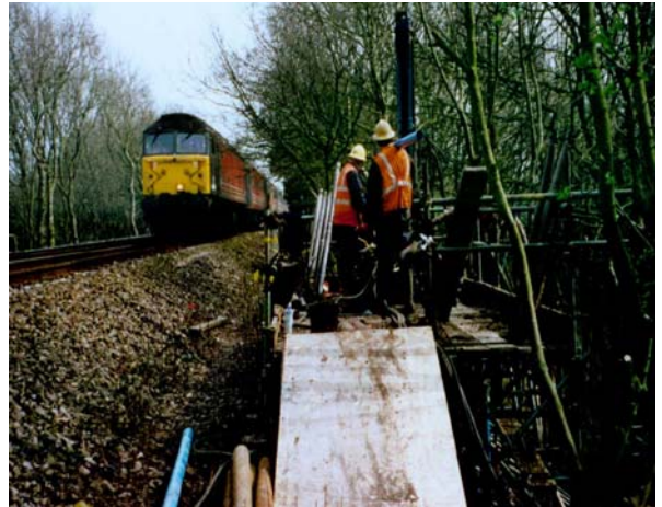
Drilling beside a railway at Coal Pit Heath, Gloucester for a Railtrack project
