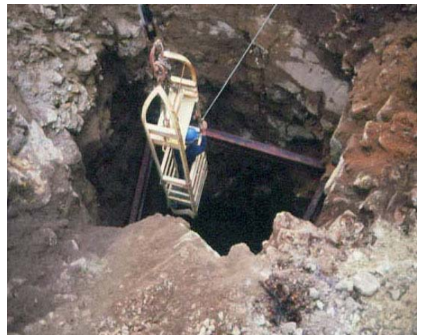
Placing steelwork for formwork for a shaft collapse scheme using a man riding basket suspended from a crane in Camborne, Cornwall
