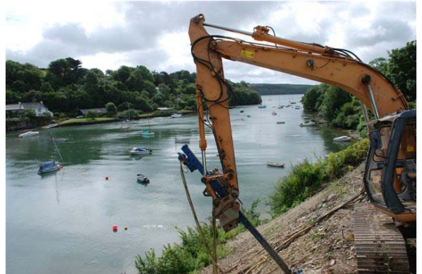
Soil Nailing the face of a Slope Failure in nr. Truro, Cornwall
