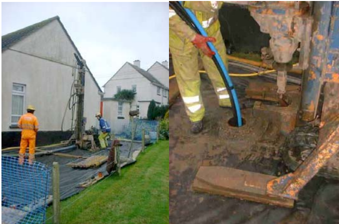
Retrofitting Domestic Properties with GSHP at Ludgvan Nr Penzance for Penwith Housing Association and Powergen
