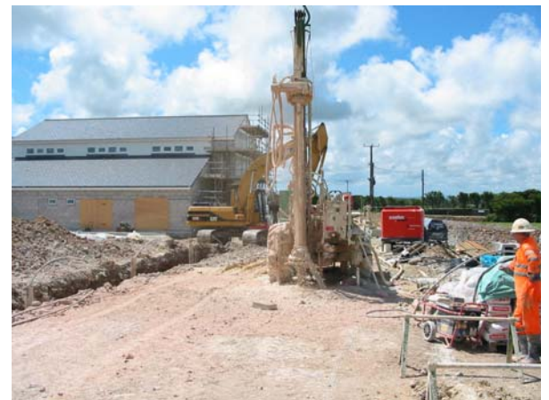
Installation of Vertical Loop Boreholes at Pencoys School, Four Lanes in Cornwall.
